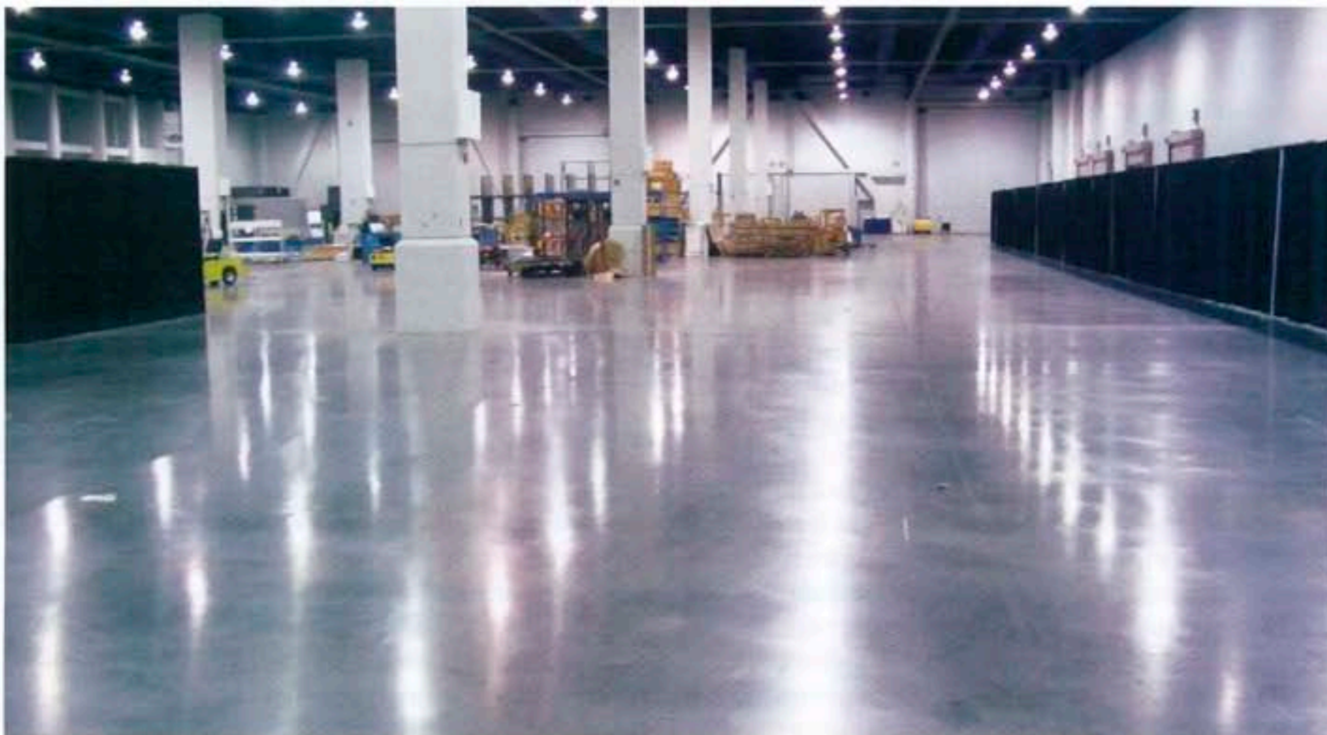
A trade fair floor compacted once with Ashford Formula after many years of use in the Las Vegas Convention Center (USA).
